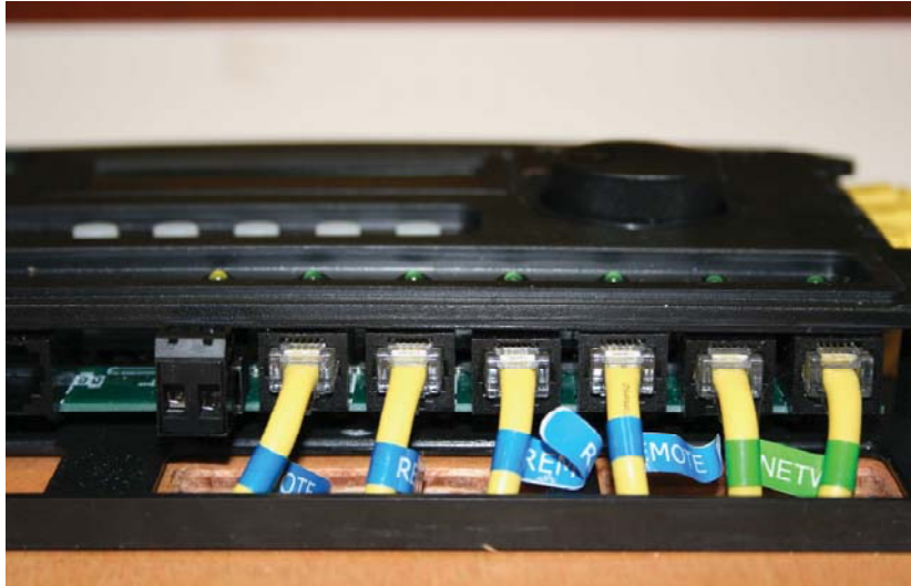
Figure 2-7, Concealed Mounted Communication Cables
